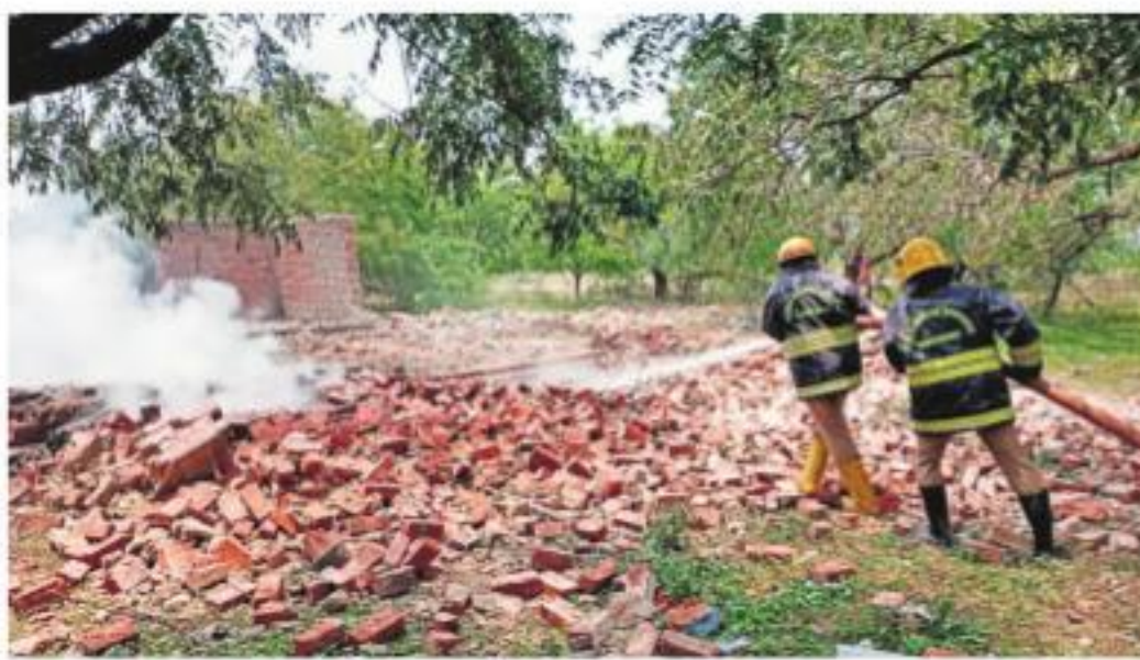
The blast location in Oorampatti, Virudhunagar district | EXPRESS
